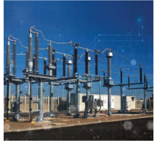
Photo Credit : HITACHI ABB POWER GRIDS
